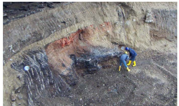
Preparing the ground: site development by specialist construction subsidiary omniCon in Munich's Arnulfpark
